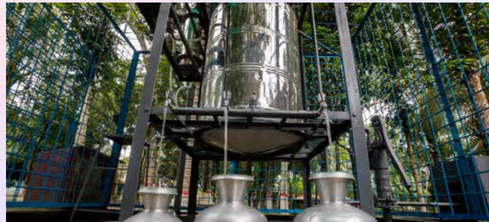
Water filtration plant at Kushtia
