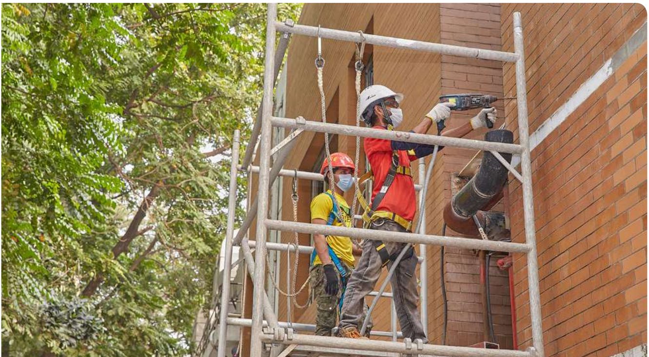
Maintenance work @ Dhaka Factory, BAT Bangladesh following all safety measures of EH&S
