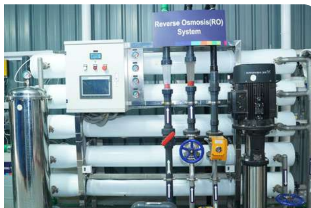
Reverse Osmosis (RO) System
