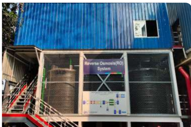
Reverse Osmosis Plant @ Dhaka Factory
