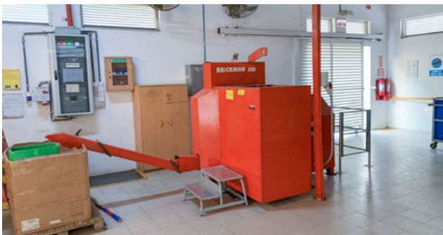
Briquette machine in briquette room
